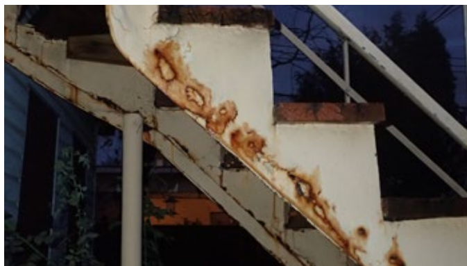
Acier corrodé – Nivoex
